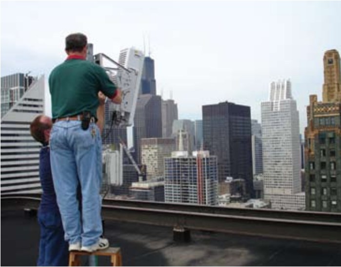
Motorola engineers install a WiMax access point on a rooftop in Chicago. Image courtesy of Motorola, Inc.
